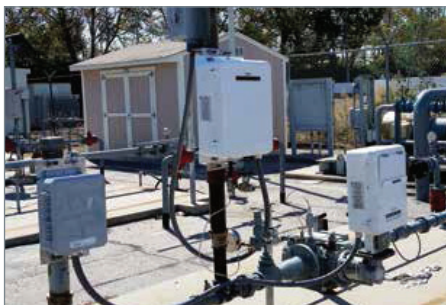
Field implementation of the Aclara pressure monitoring solution with transmitter at far left and pressure monitor at far right.
